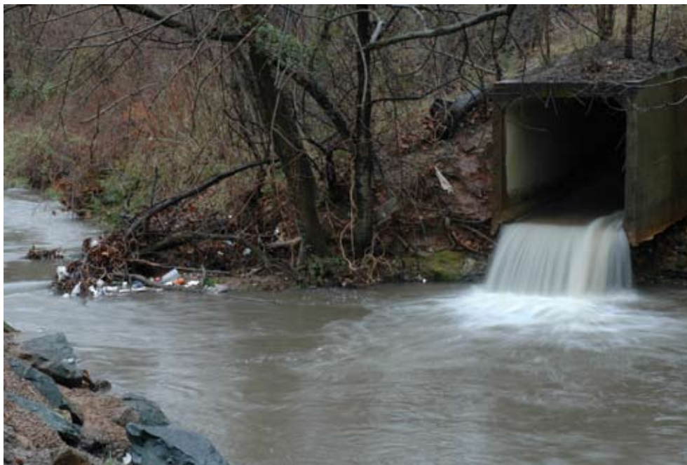
Stormwater runoff flows directly into Schenks Branch near the intersection of McIntire Road and Harris Street.
