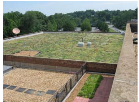
A good example of a green roof can be found on the Albemarle County office building located on McIntire Road in the City.
